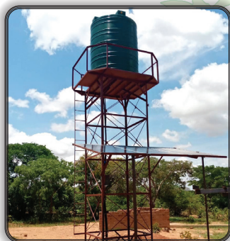
Solar water pump
